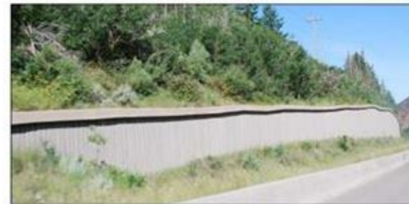
E | Structural retaining devices should be utilized to stay within the existing limits of disturbance.
